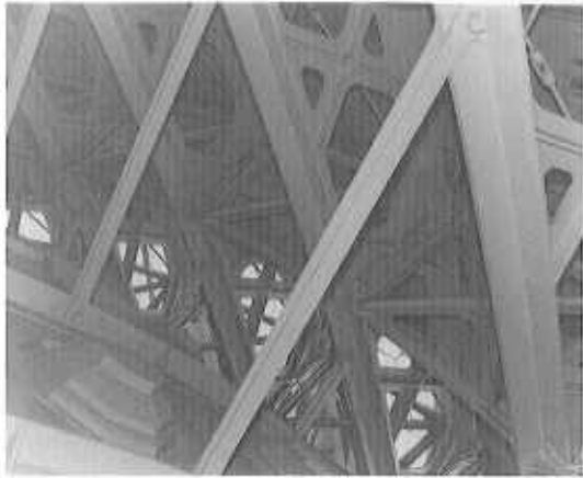
Cast-iron interior framing of ribs and circumferential bracing in U.S. Capitol dome. Courtesy National Museum of American History, Smithsonian Institution.
