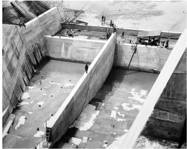
The “hydraulic jump,” featuring a series of steps and a wall to hold a pool, was one of the water calming innovations developed by Conservancy engineers. Photo courtesy Wright State University
